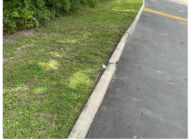
Concrete curb cracks
