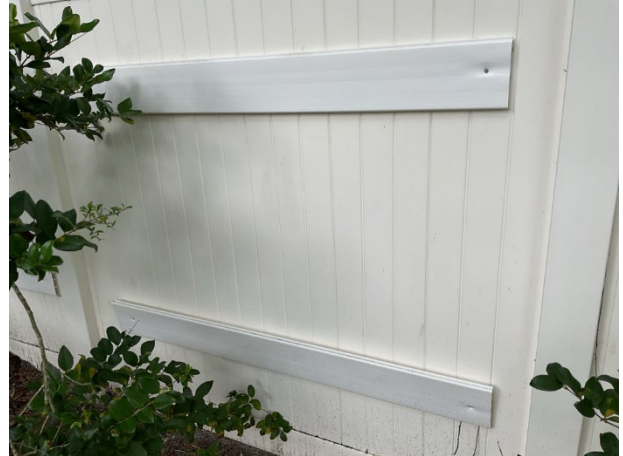
Vinyl fence previous repairs
