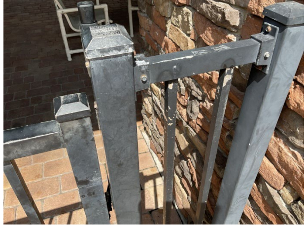
Fence finish deterioration
