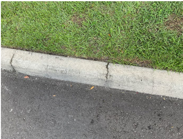
Concrete curb cracks
