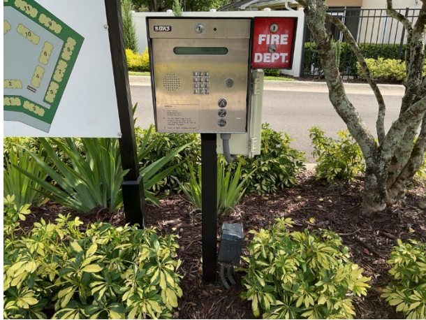
Gate entry keypad
