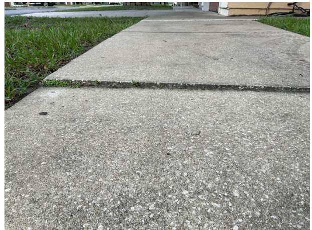
Sidewalk trip hazard
