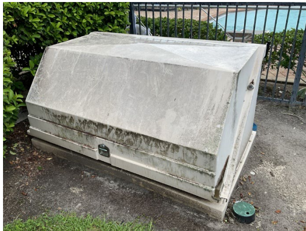
Pool mechanical equipment enclosure
