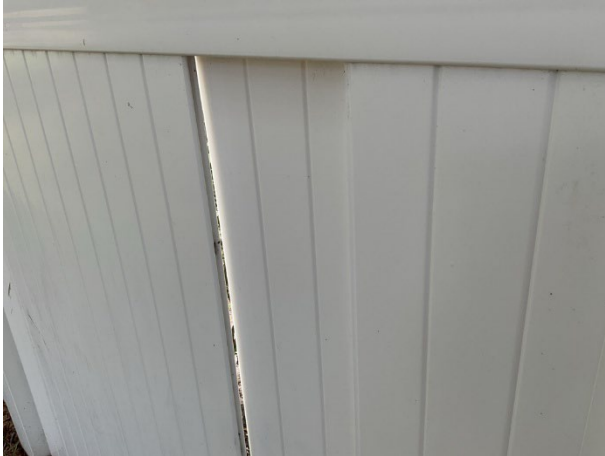
Fence dislodged section
