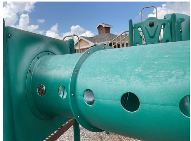
Equipment finish deterioration
