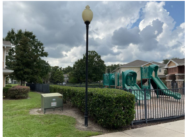
Light pole and fixture
